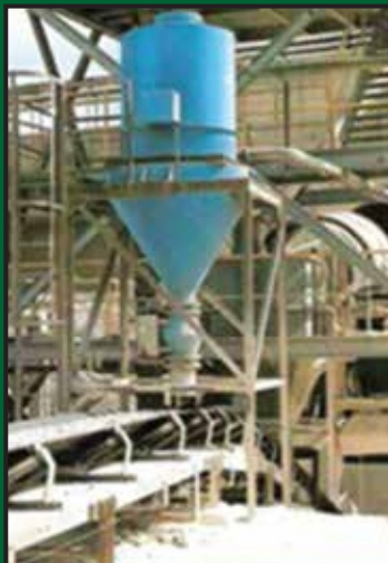
INTERCEPT CYCLONIC HOPPER DIS-CHARGING ON CONVEYOR FO RE-CYCLE.
